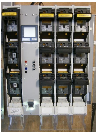
BBS6 with internal MDI & phasing sockets & streetlight fuse carrier.
