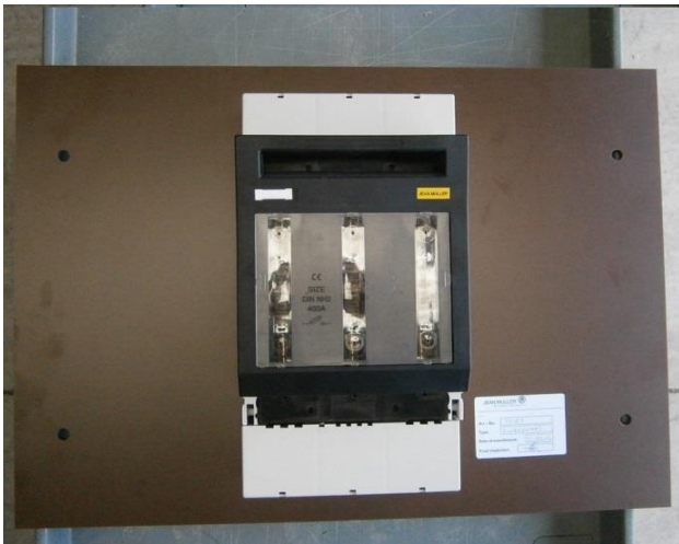
200KVA tx 1 x LTL2-3 400 amp
