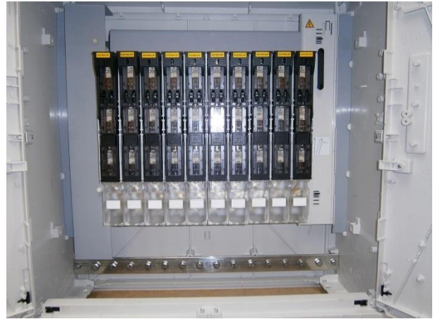
KVS1 with SL00/100 fuse switches for a poultry shed complex & mounted direct to a concrete base.
