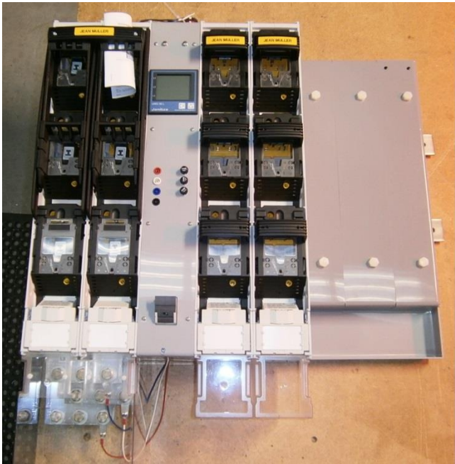
BBS8-1300IUMG with 1250 amp isolator, internal MDI, Phasing sockets, street light fuse carrier at the bottom & 3 spare 100mm ways.
