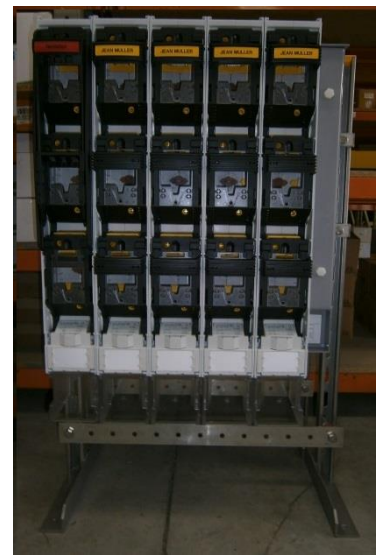
6 way Free standing LV rack with 1 spare 100mm way & N/E bar.
