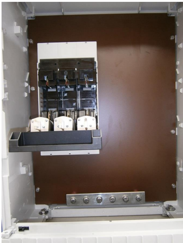
KVS00 with formica panel LTL2 400amp fuse switch & N/E bar
