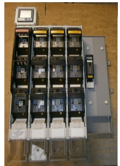
BBS6 with top MDI, 1-pole Street light disconnect & 1 spare 100mm way.
